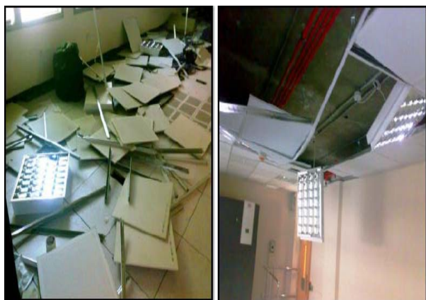
Figure 2. Colapse of the suspended ceiling
