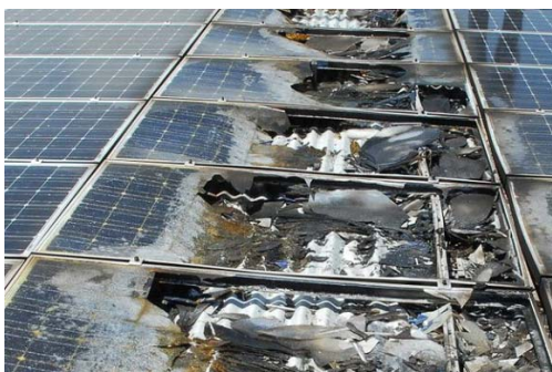
Figure 4. Third case - fire begins from photovoltaic equipment
