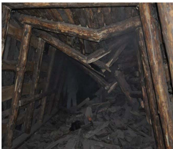
Figure 3. Collapsed ventilation hall of the mine pit
