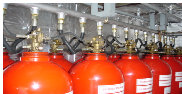
Figure 1. Fixed fire suppression system [4]
