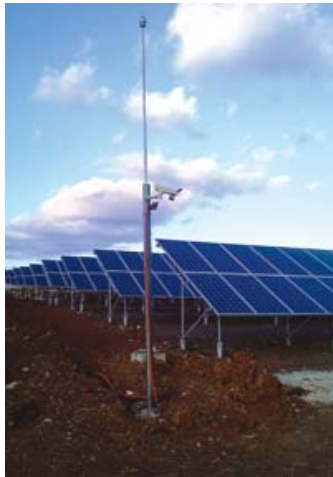
Figure 8. Outside lightning protection
