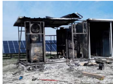
Figure 9. Fire in transformer inverter station
