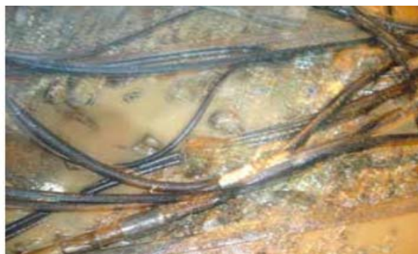
Figure 4. Electricity distribution as a cause of higher risk [3]
